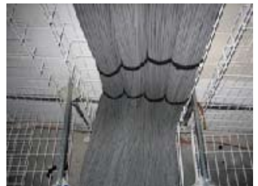
Image: Shielded cabling maintains signal integrity. Large cable bundles are common in Data Centres
